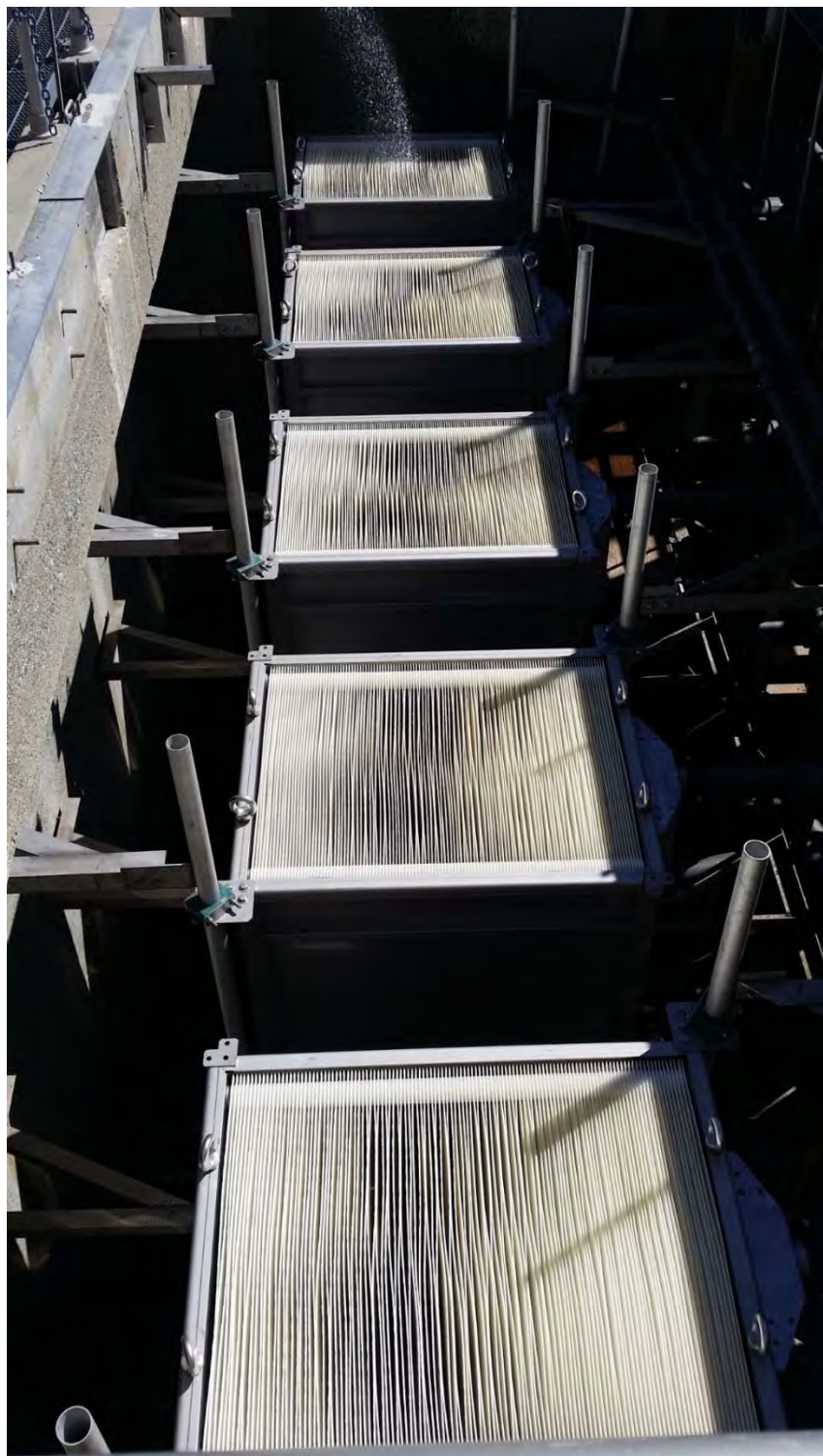
Five Ovivo OV960 SMU's Installed at RSWD WWTP
