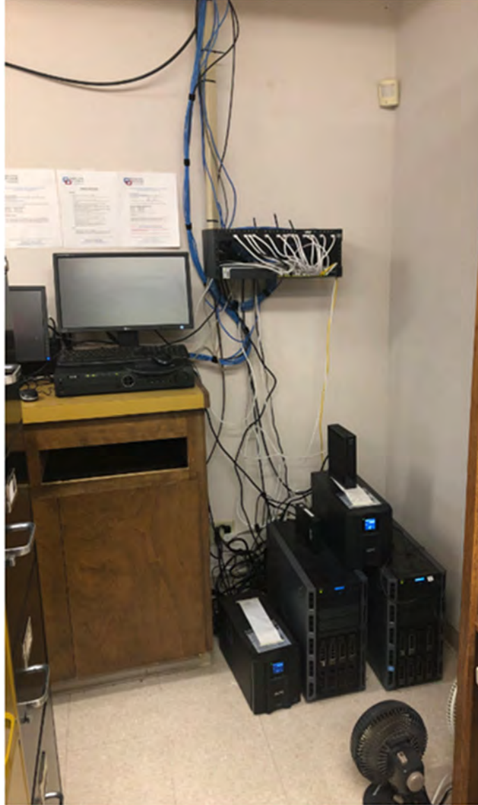
Existing Server Room Configuration
