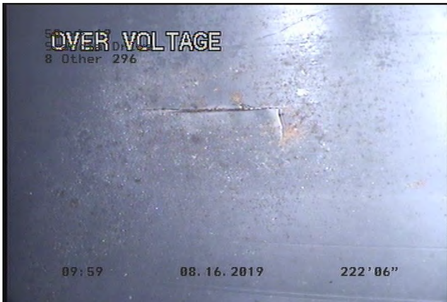
Photo: 50-19-CL-16.JPG 222.48FT, Crack Longitudinal, at 01 o'clock, within 8 inches of joint: NO
