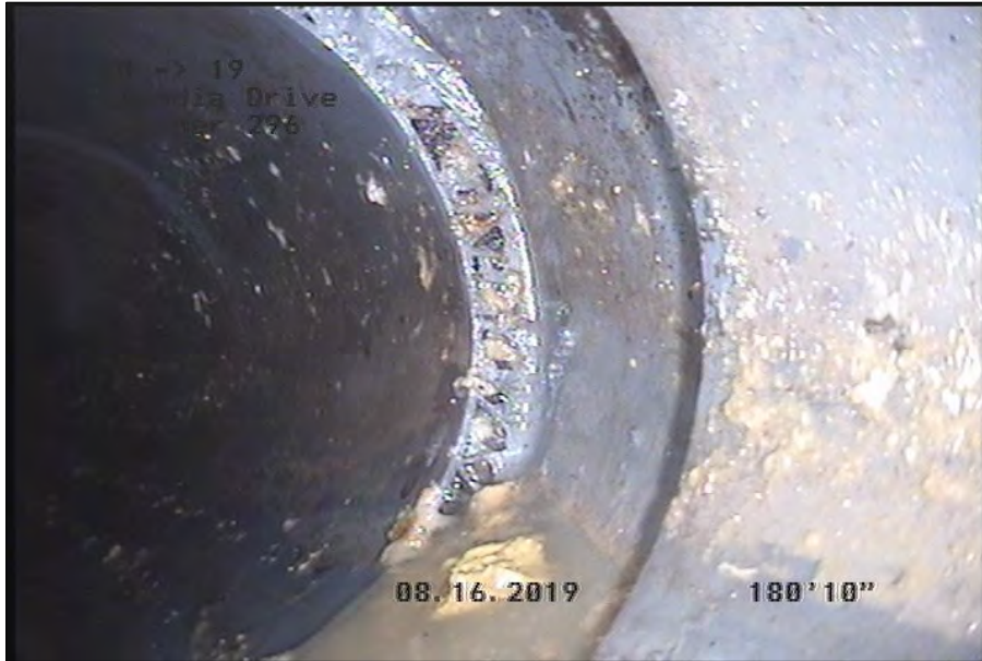
Photo: 50-19-JSL-15.JPG 180.87FT, Joint Separated Large
