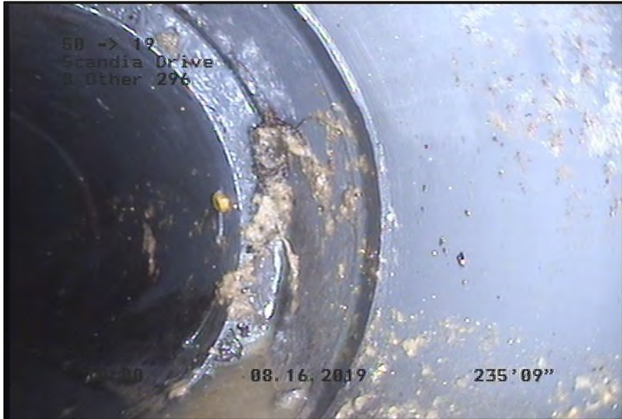
Photo: 50-19-JSL-17.JPG 235.72FT, Joint Separated Large
