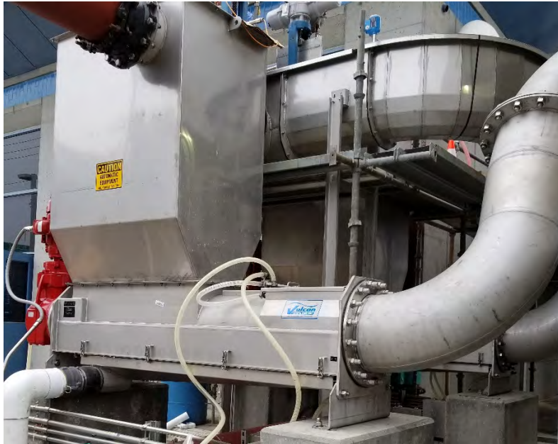
Washing Press with sluice trough inlet hopper shown.
