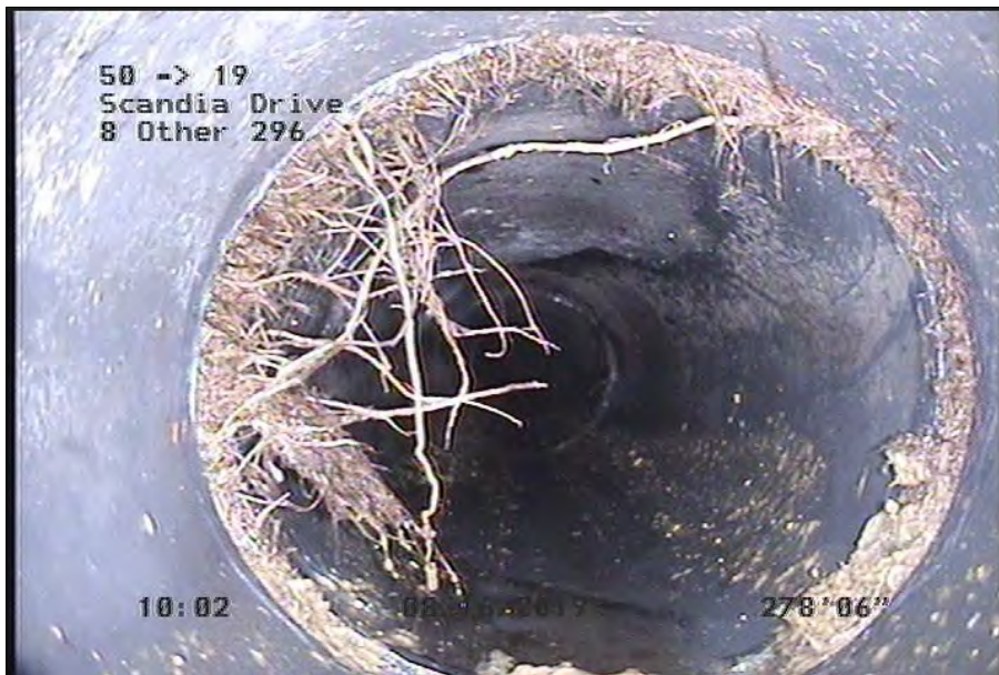
Photo: 50-19-RFJ-19.JPG 278.53FT, Roots Fine Joint, from 12 to 12 o'clock, within 8 inches of joint: YES
