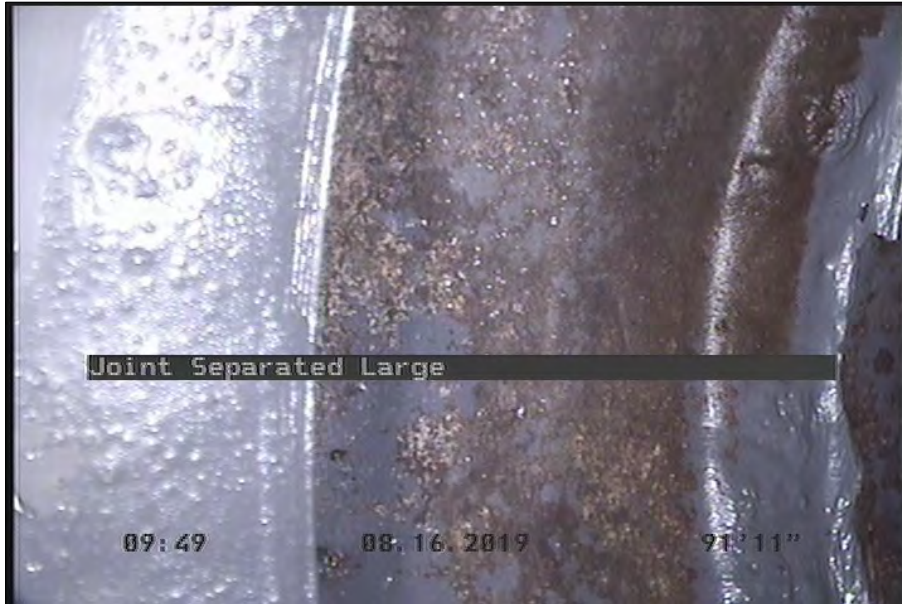
Photo: 50-19-JSL-9.JPG 91.94FT, Joint Separated Large
