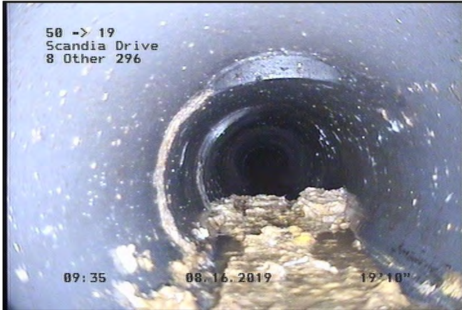
Photo: 50-19-DAR-4.JPG 19.85FT, Deposits Attached Ragging, 10 %of cross sectional area, from 05 to 07 o'clock, , within 8 inches of joint: YES
