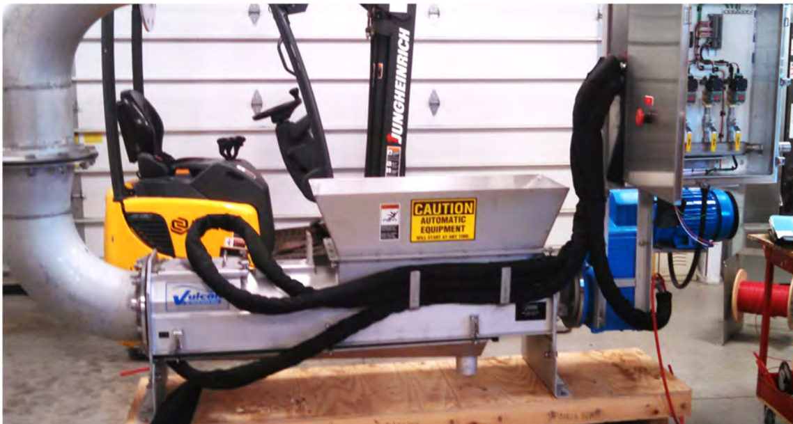
Washing Press with heat traced water lines.
