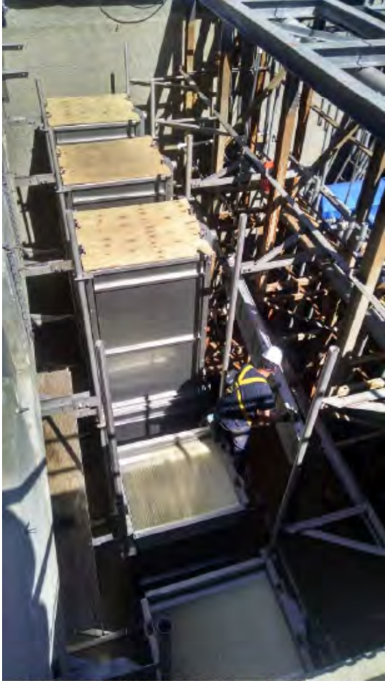
Five Ovivo OV960 SMU Installation at R5WD WWTP
